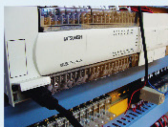
Japan, Mitsubishi PLC system
